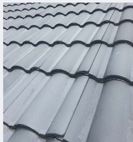
Does your roof appear faded or dull? Environmental fallout such as salt residue, dirt or dust deposits can cause this aesthetic change.
